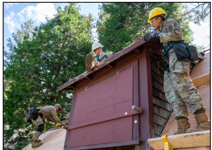
U.S. Air Force Airmen from the 152nd Civil Engineer Squadron work to restore a shake roof on a cabin at Tallac Historic Site, South Lake Tahoe, Calif., September 11, 2023. The 152nd Civil Engineer Squadron has been working on historical restoration construction projects at Tallac Historic Site since 1983.
