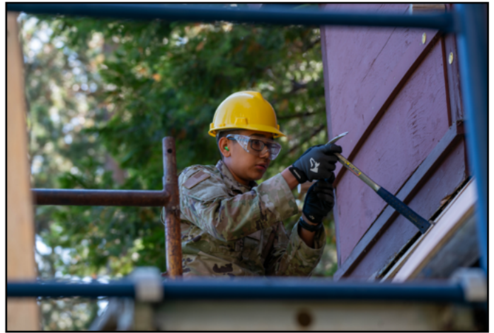
U.S. Air Force Airman 1st Class Adan Albarran Ayala, 152nd Civil Engineer Squadron structural specialist, uses a hammer to help restore a shake roof at Tallac Historic Site, South Lake Tahoe, Calif., September 11, 2023. The 152nd Civil Engineer Squadron has been working on historical restoration construction projects at Tallac Historic Site since 1983.
